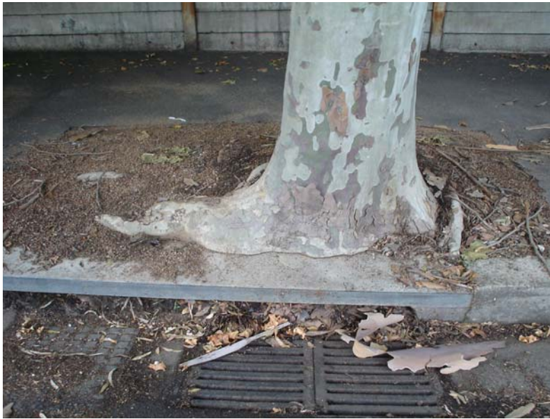
Photograph 1: Illustrating the conflicts between trees and infrastructure in a number of trees on the Wilson Street frontage of the site.
